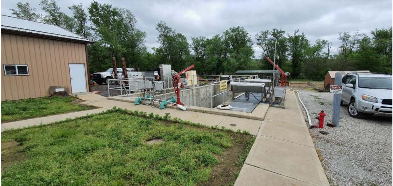
Figure 3-8 - Disinfection & Post Aeration Structure
