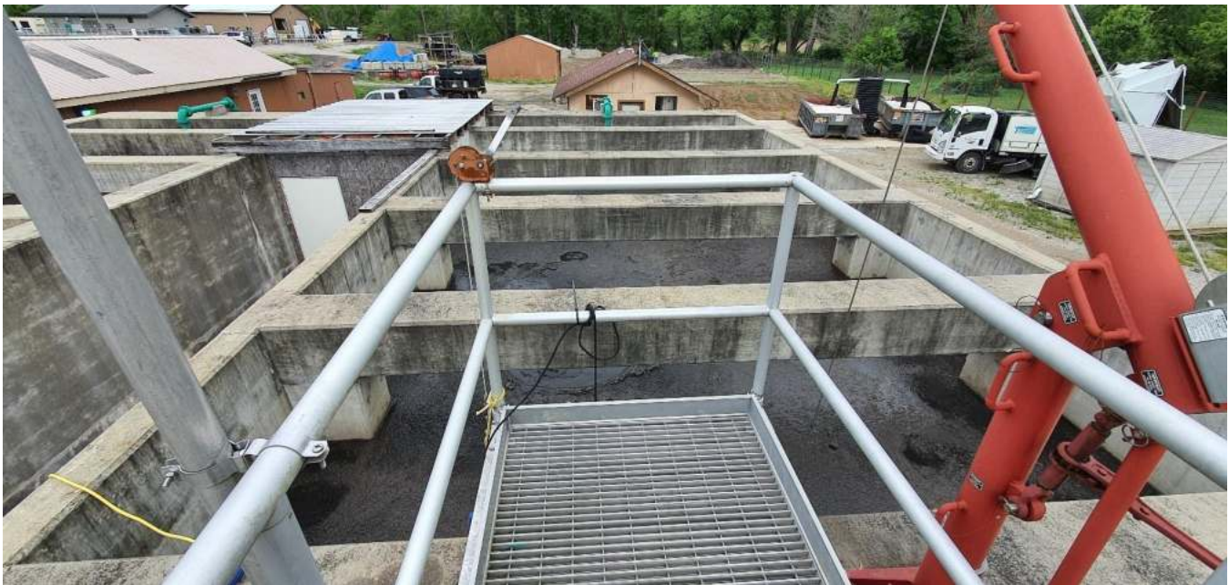
Figure 3-11- Aerobic Digester Tankage
