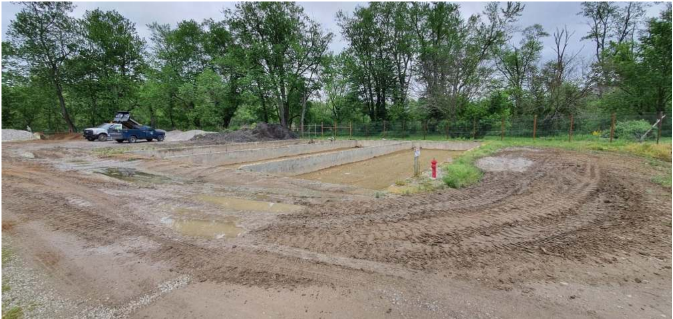
Figure 3-12- Sludge Dewatering Beds
