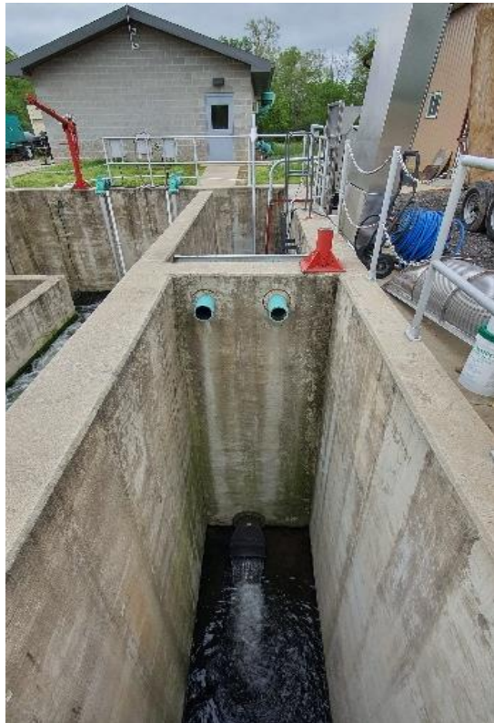
Final discharge basin w/ effluent pumps
