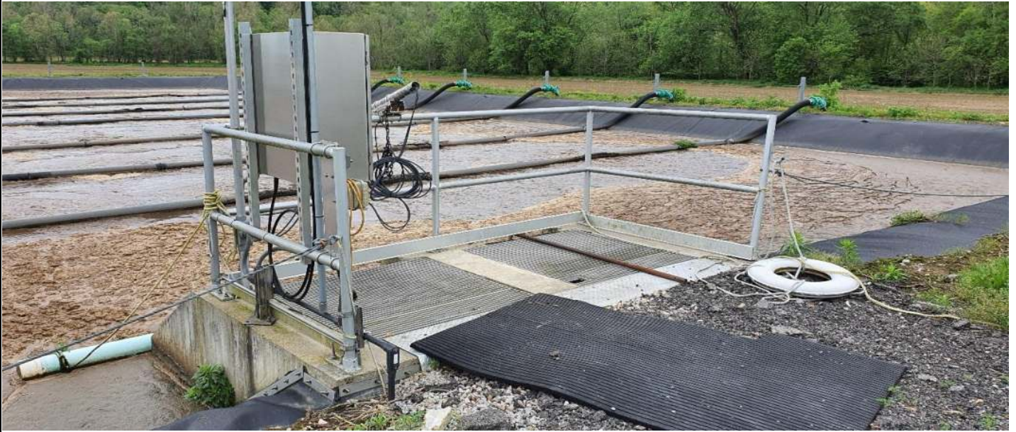
Aerated Lagoon - Effluent Structure
