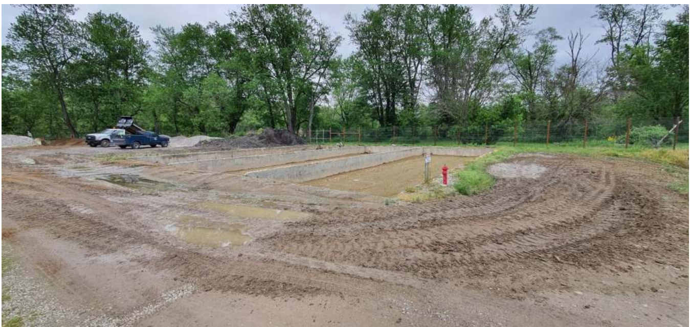
Figure 3-12- Sludge Dewatering Beds
