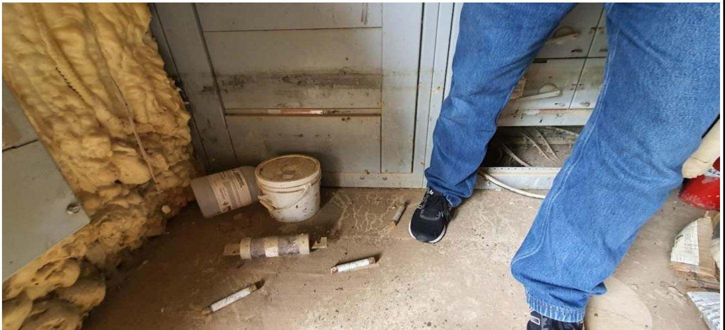
Chemical Storage Building - Decommissioned Electrical w/ Flood Damage
