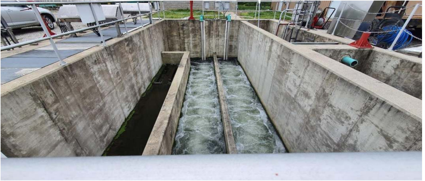
Post Aeration Tank w/ Non-potable Water System
