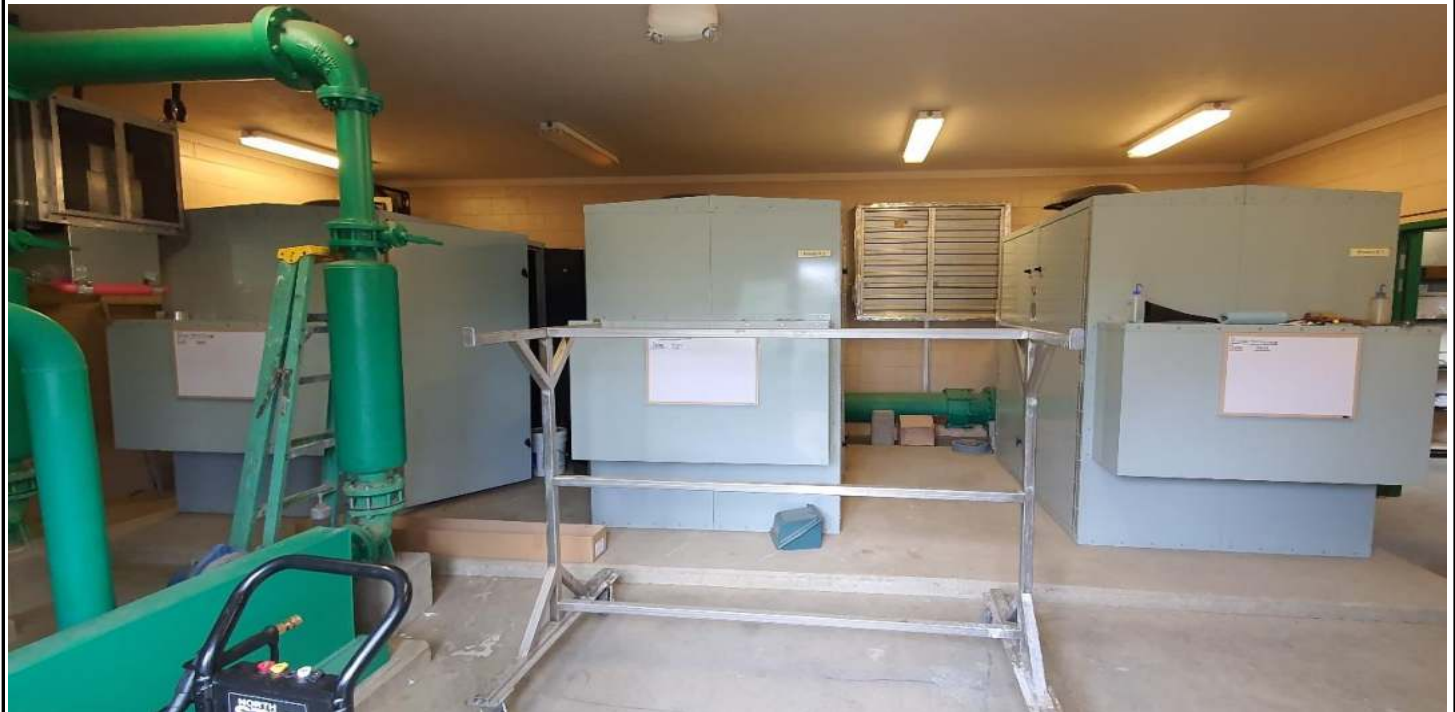
Blower Building - Blower Room
