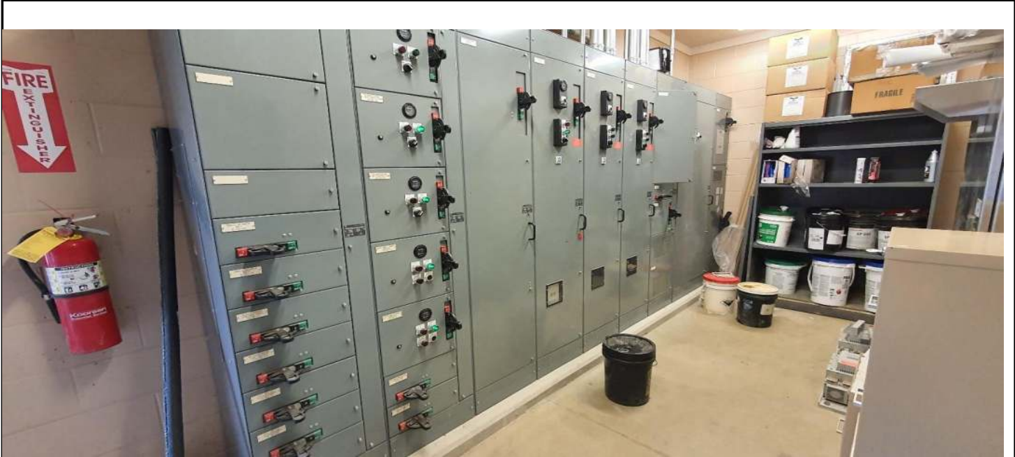
Blower Building - Electrical Control Room
